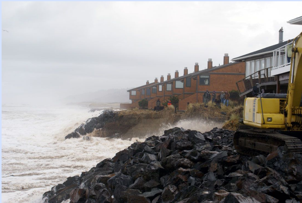
Figure 6.14. Loss of beach at Neskowin has increased the potential for waves to damage coastal structures built to protect properties as well as increased the potential for flooding of homes built behind the structures.
